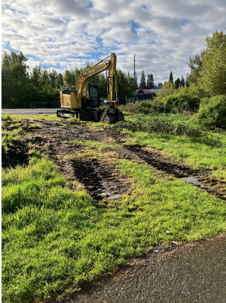
Photo 10 – April 16, 2026 – Removal Path & Damage
