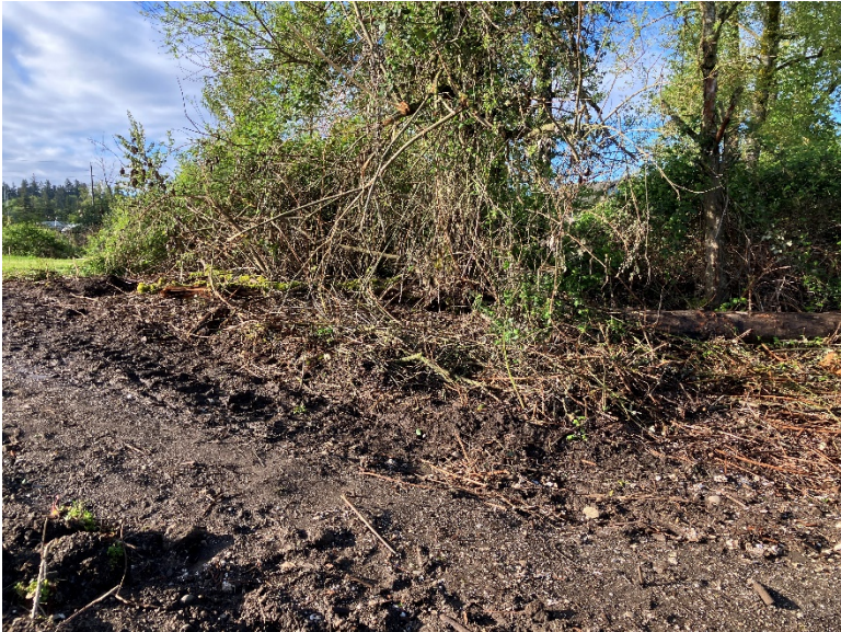
Photo 18 – April 16, 2026 – Removal Path & Damage
