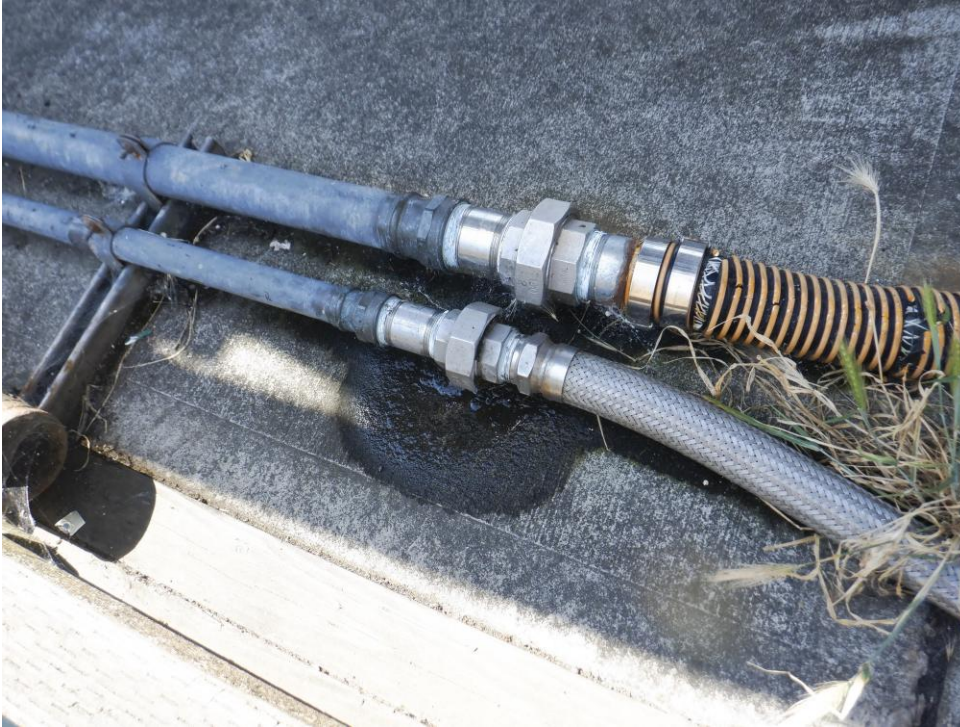
Figure 5: Leaking utilities, located beneath ramp.
