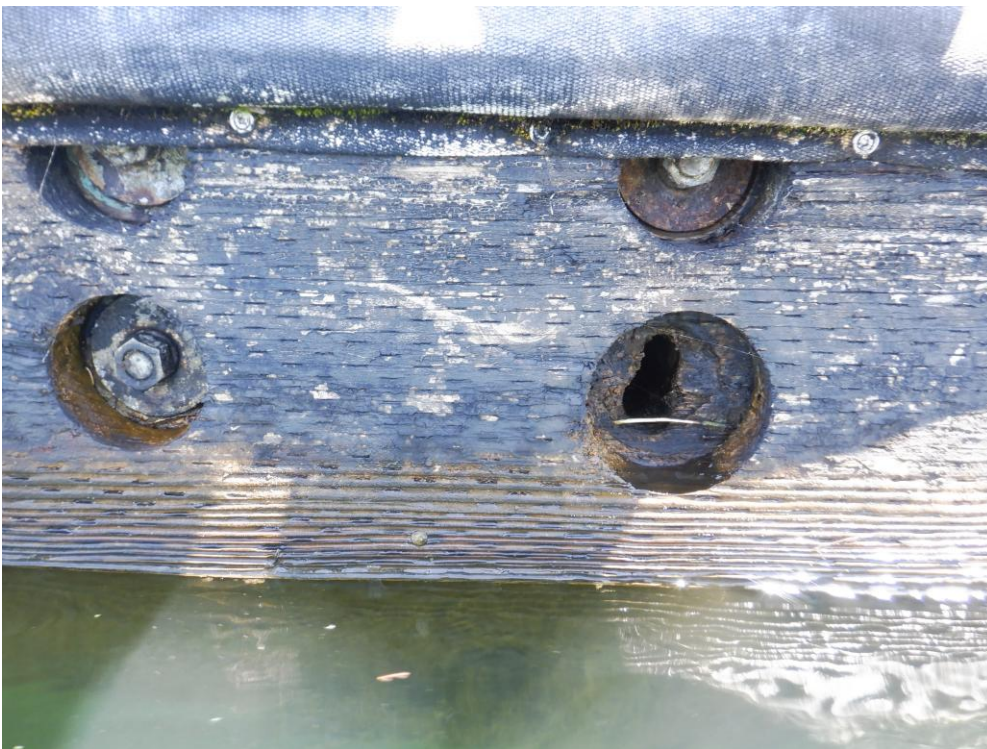
Figure 10: Missing tie rod at float section 9 from North end of dock.
