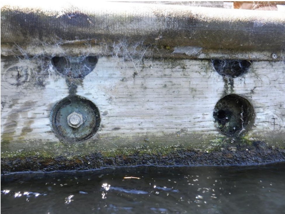
Figure 2: Missing bolts observed in fender system.
