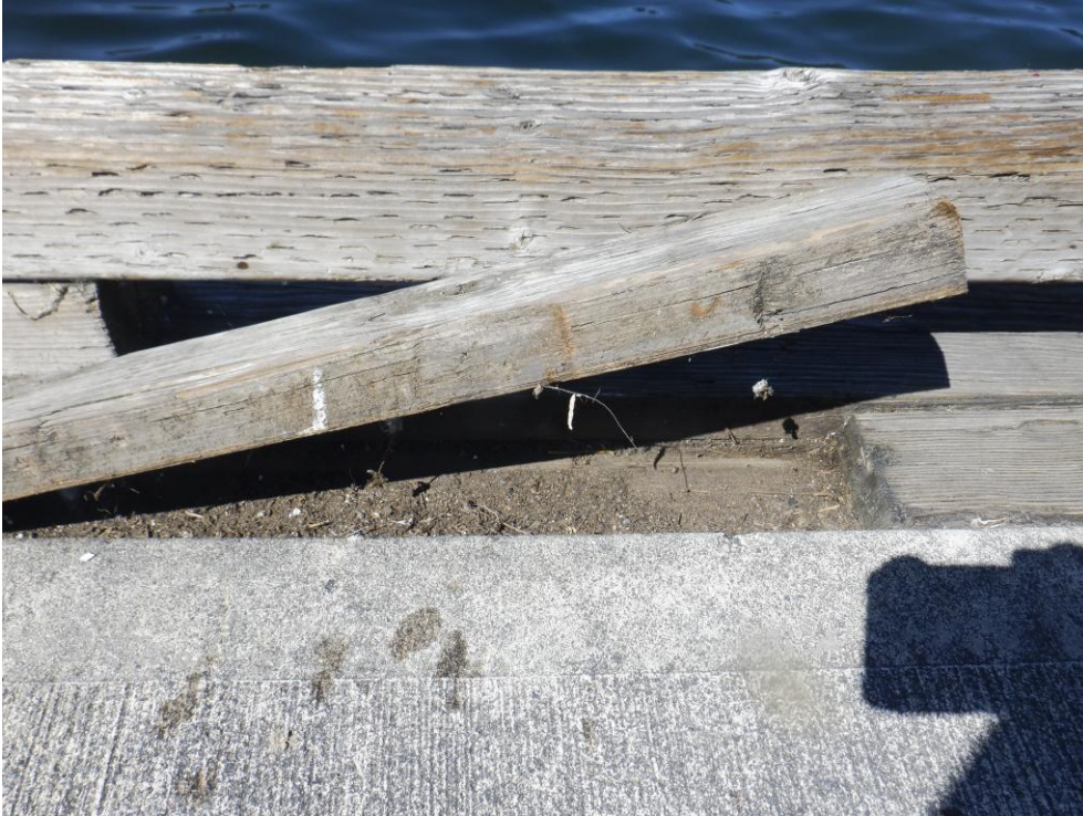
Figure 3: Detached timber section along fender system.
