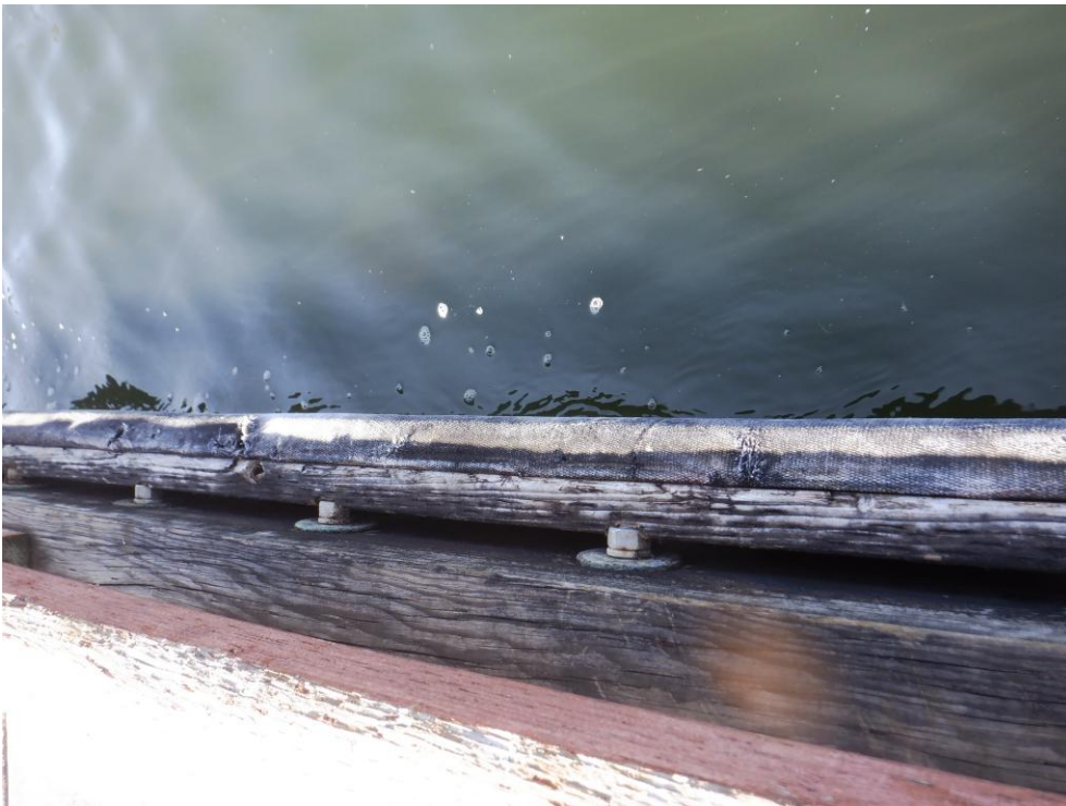
Figure 4: Broken timber fender section.
