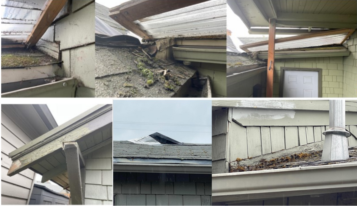
Figure 6 Roof design and disrepair
