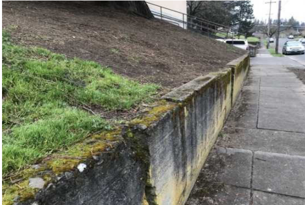
43 LEANING RETAINING WALL
