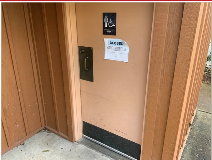
2 – ENTRANCE DOOR HARDWARE
