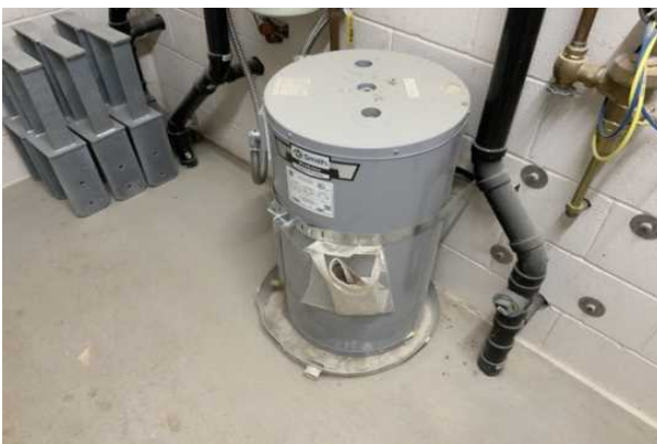
15 WATER HEATER, ELECTRIC
