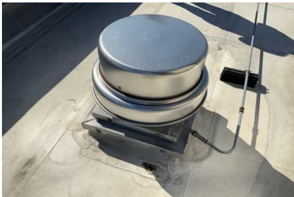
27 ROOF-MOUNTED EXHAUST FAN
