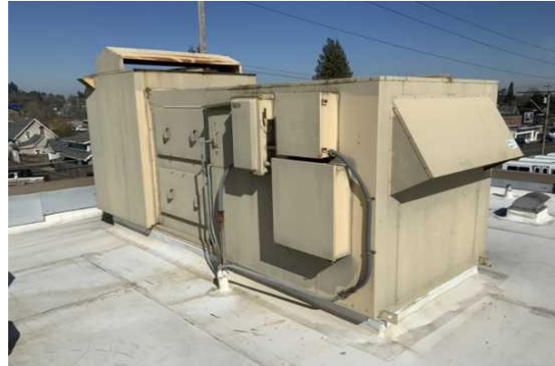
26 MAKE-UP AIR UNIT
