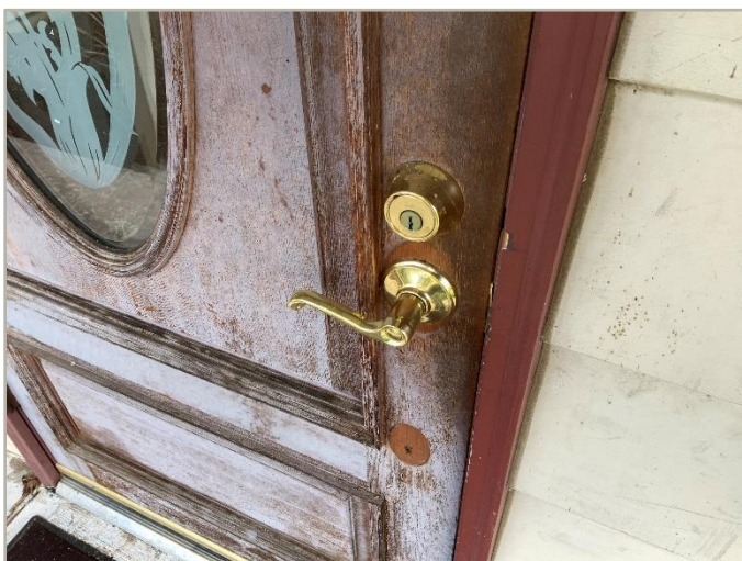
3 – ENTRANCE DOOR HARDWARE
