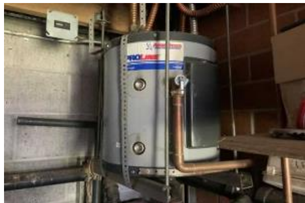
12 WATER HEATER, ELECTRIC
