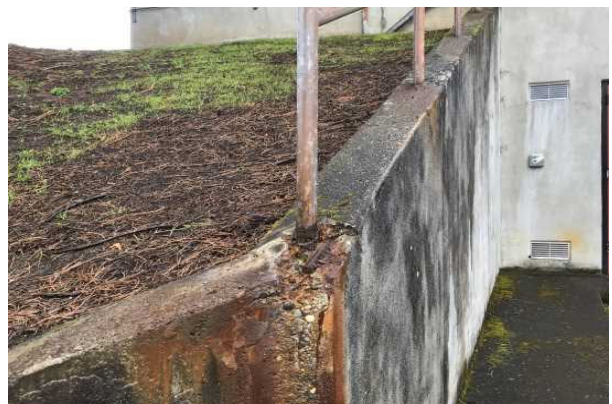
46 RETAINING WALL SPALLING
