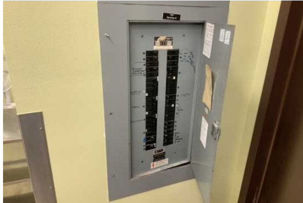
31 MAIN DISTRIBUTION PANEL
