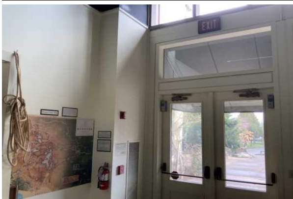
35 FIRE ALARM SYSTEM
