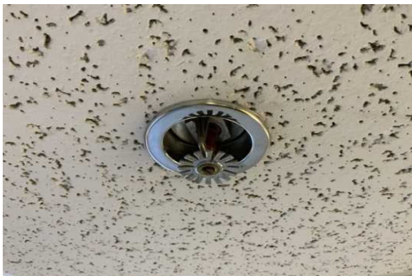
29 FIRE SPRINKLER SUPPRESSION SYSTEM
