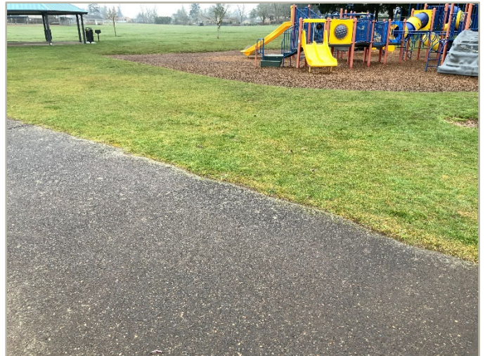
10 – LACK OF ACCESSIBLE ROUTE TO PLAYGROUND
