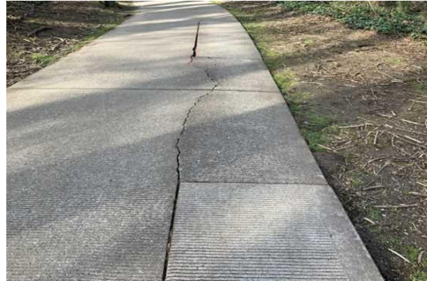
8 SIDEWALK, CONCRETE, LARGE AREA
