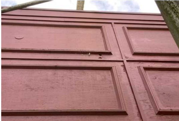
7 DAMAGED EXTERIOR WOOD WALL
