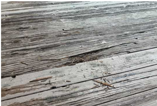
9 ROTTING WOOD DECKING
