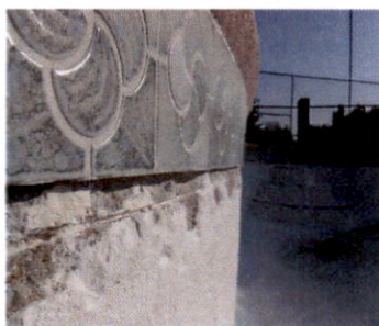
Saw-cut and chip below tile
