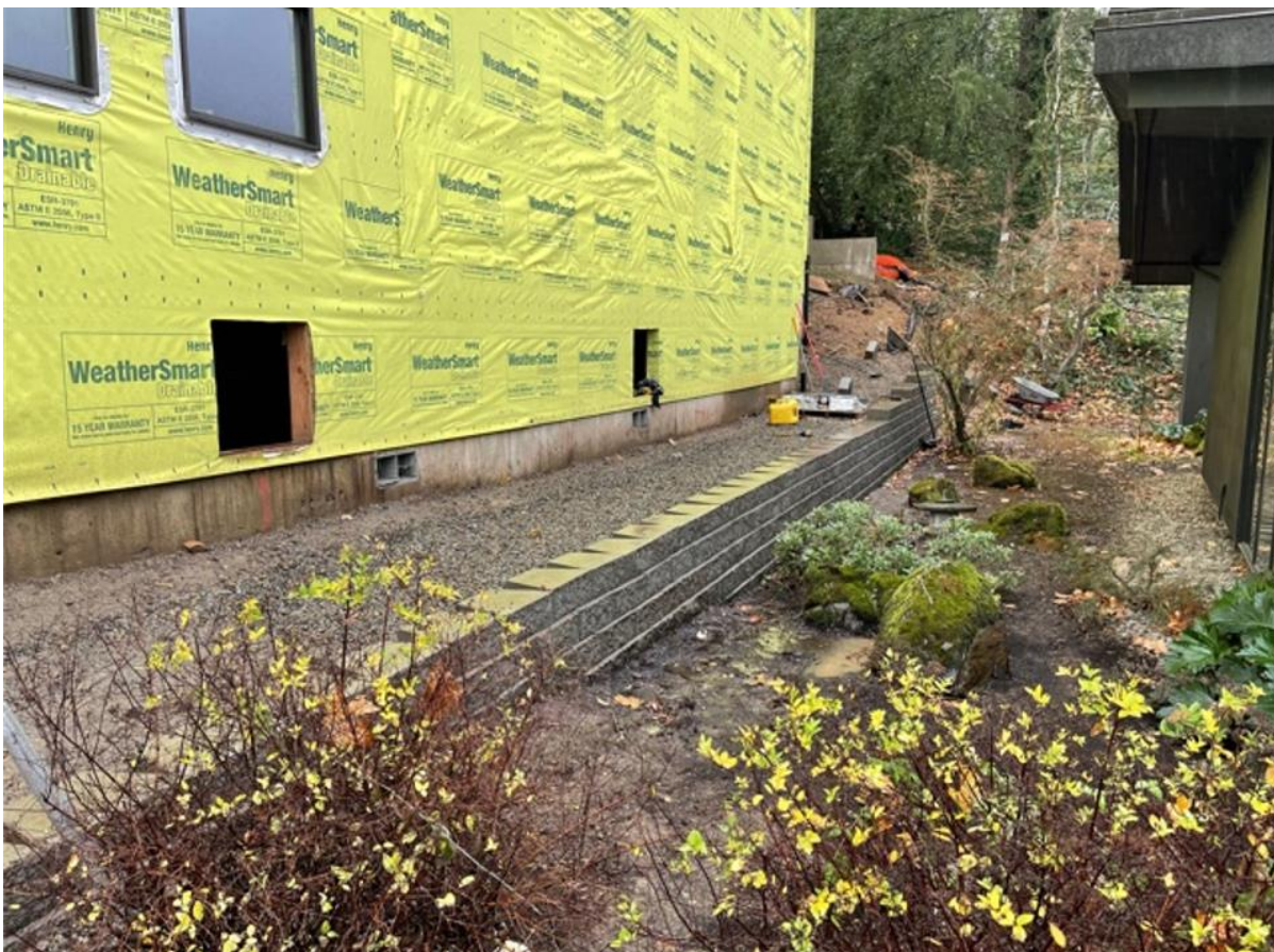
Figure 12- Side elevation photo (submitted 11.15.21) showing unpermitted retaining wall
