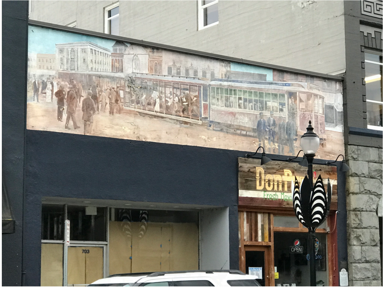
The state of the mural before restoration
