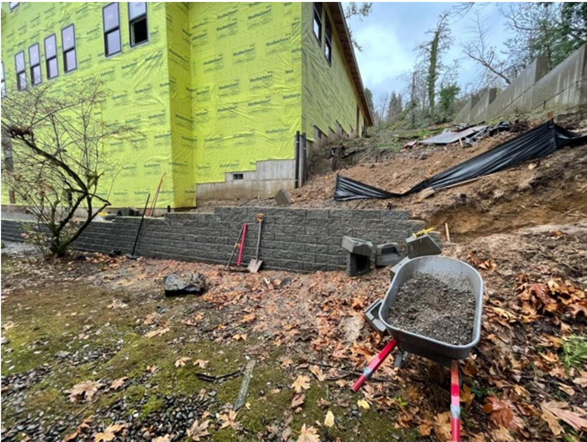
Figure 11- Side and rear elevation photo (submitted 11.15.21)- showing unpermitted retaining wall
