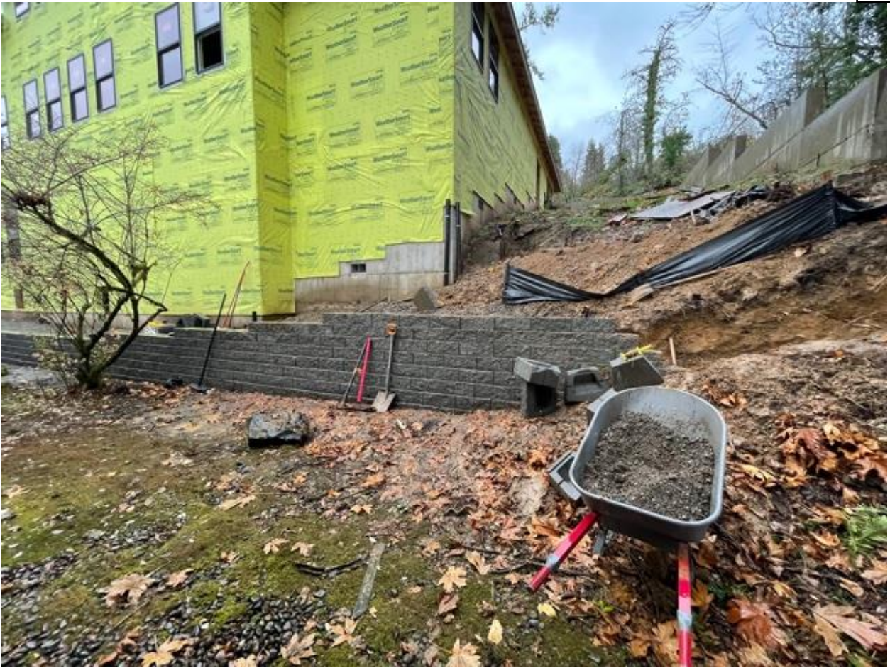
Figure 5 Existing condition showing unpermitted CMU wall. Provided in 11.15.21 Applicant's resubmittal. The CMU wall does not meet Conditions of Approval 3 and 7 of HR 20-01 and will need to be rebuilt using poured in place concrete, basalt veneer, or natural rockery.
