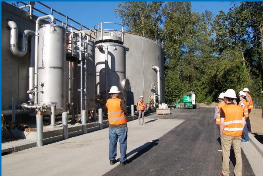
WES Advisory Committee members tour the digester complex.
