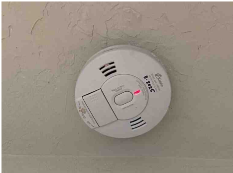
Smoke/Co Det Sample
