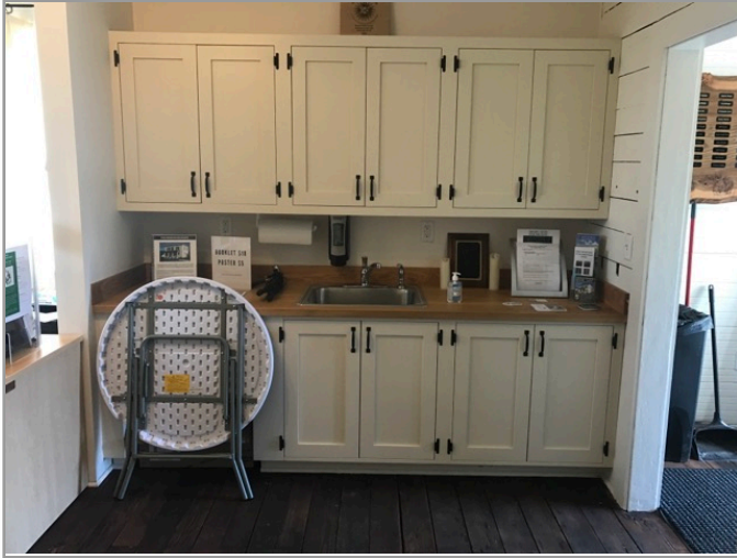
Kitchen cabinets/sink clearance
