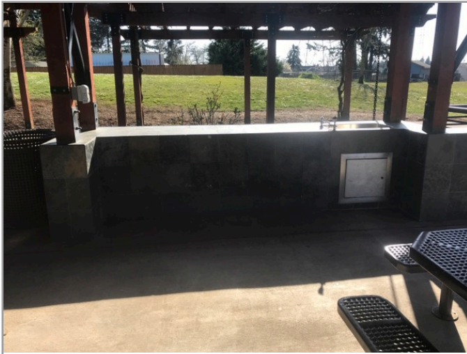
Kitchen cabinets/sink clearance
