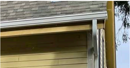
Fascia - Permitted / As Built
