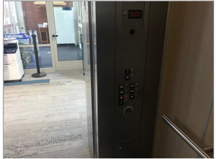
In-cab controls/emergency call panel
