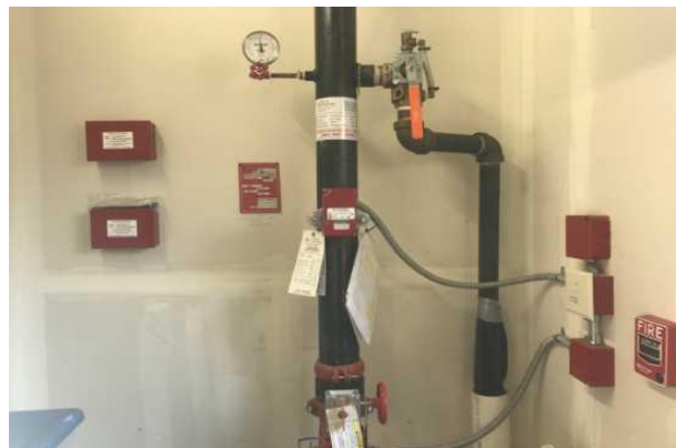
18 FIRE SUPPRESSION SYSTEM
