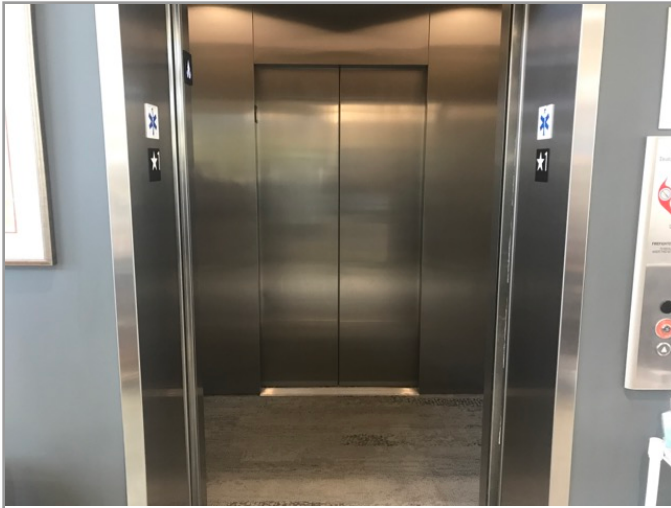
Lobby looking at cabs (with doors open)
