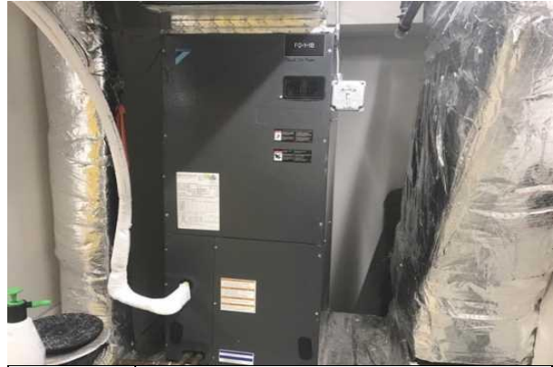
14 SPLIT SYSTEM FAN COIL UNIT
