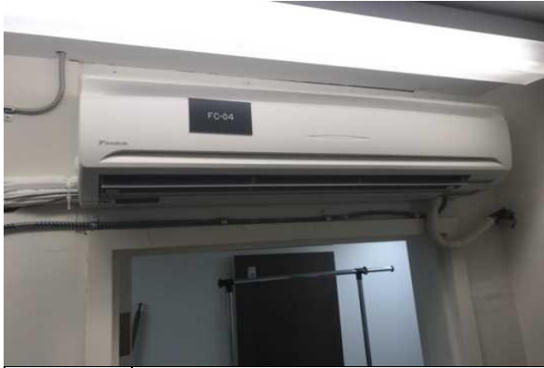
13 SPLIT SYSTEM FAN COIL UNIT
