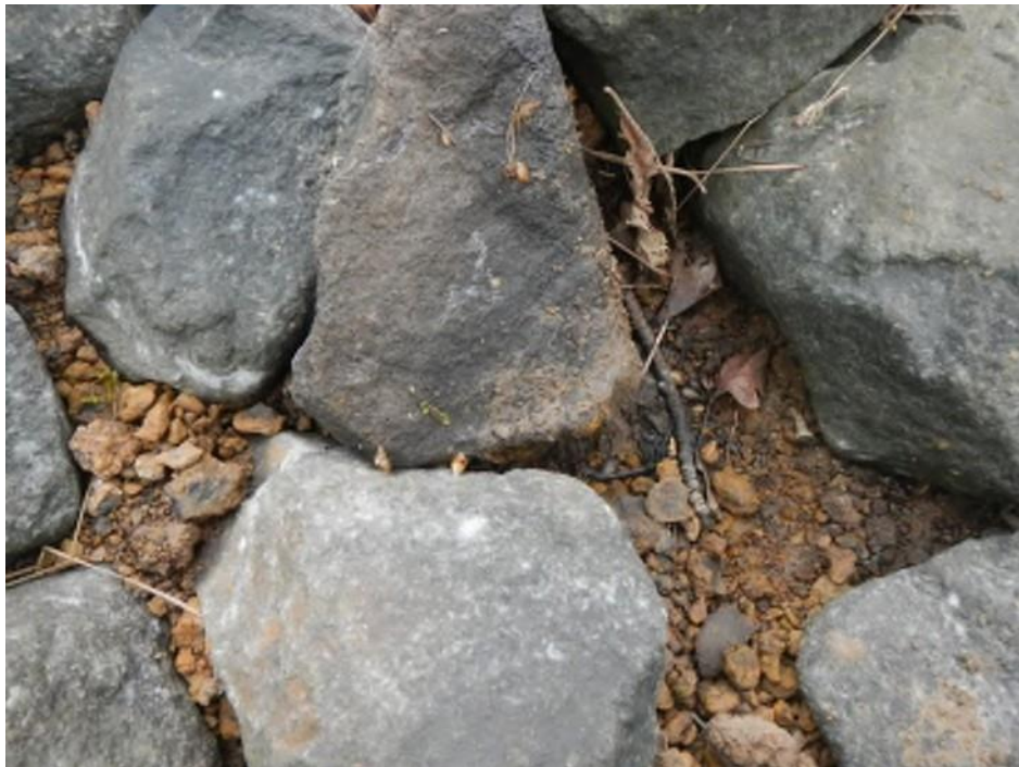
Photo 8. Aquatic snail shells are present amongst riprap in the pool area of the culvert inlet.
