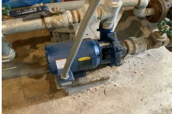
14 PUMP, DOMESTIC WATER
