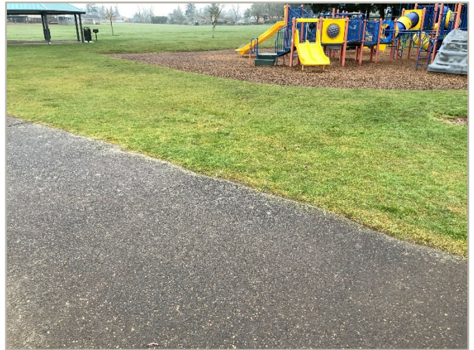
10 - LACK OF ACCESSIBLE ROUTE TO PLAYGROUND
