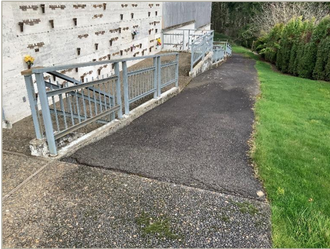
3 - EXTERIOR RAMP MISSING RAILINGS
