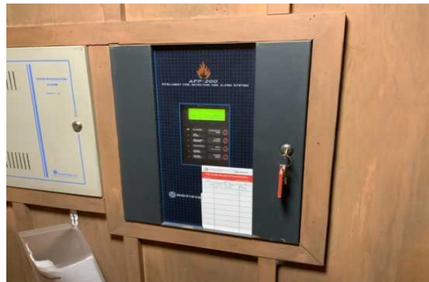
34 FIRE ALARM CONTROL PANEL
