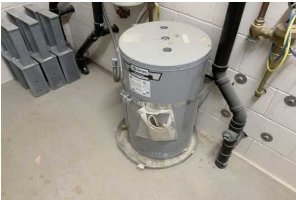
15 WATER HEATER, ELECTRIC
