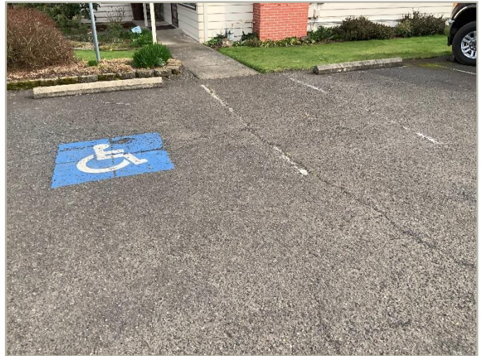
2 - MISSING ADJACENT AISLE STRIPING
