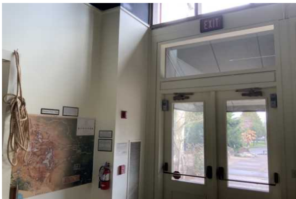
35 FIRE ALARM SYSTEM
