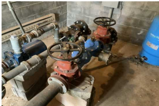
16 BACKFLOW PREVENTER, DOMESTIC WATER
