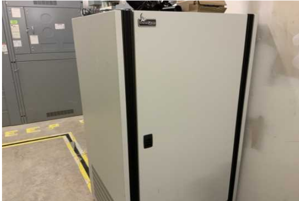
31 EMERGENCY UPS SYSTEM
