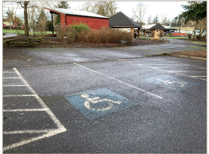
2 - MISSING PARKING SIGNAGE
