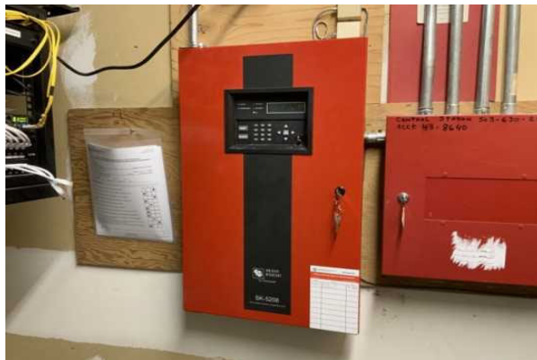
33 FIRE ALARM CONTROL PANEL
