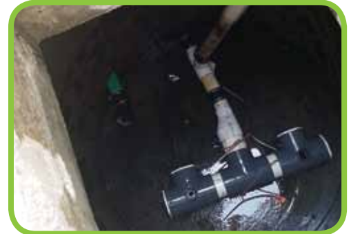
Manifold Tee View of a Cleaned System
