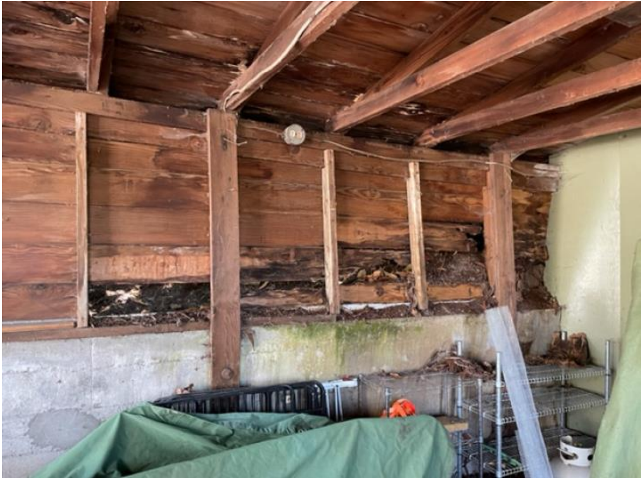
Carport wall deterioration
