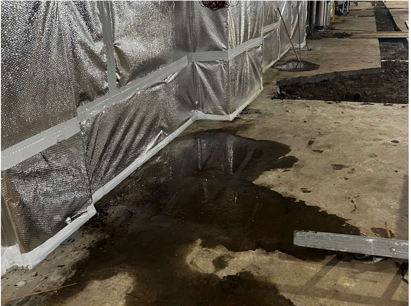
Water intrusion into basement
