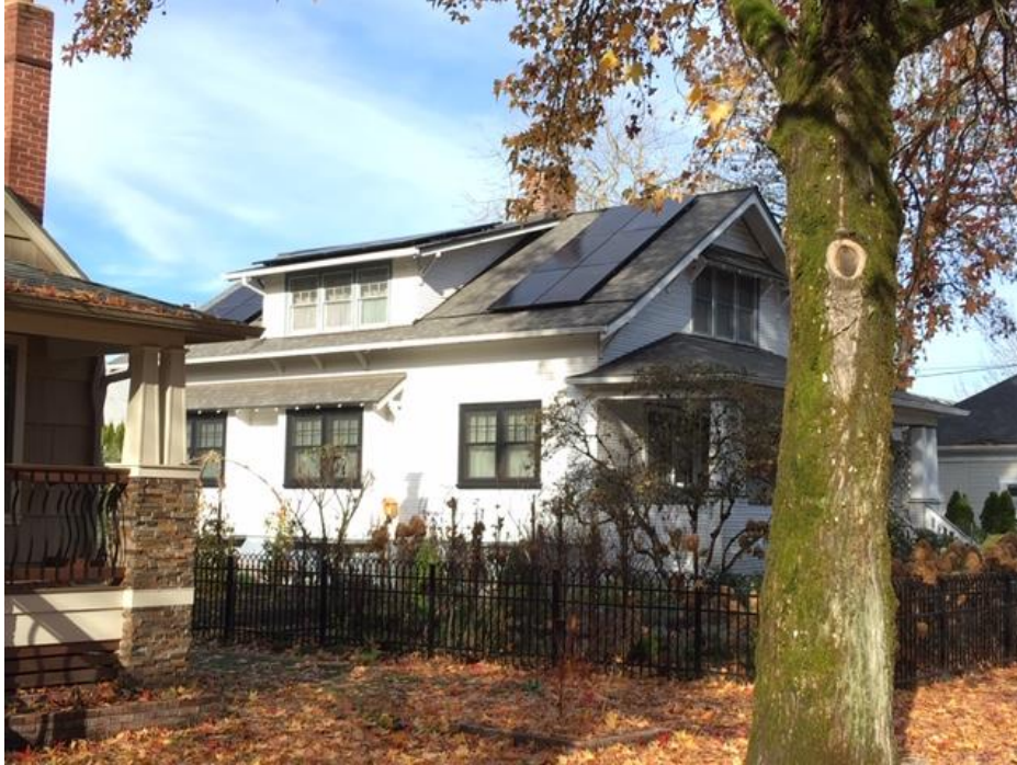
Panels on a home on Washington Street
