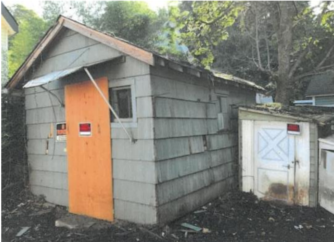
Existing Conditions- rear storage shed- identified as deteriorated contributing in survey form.
