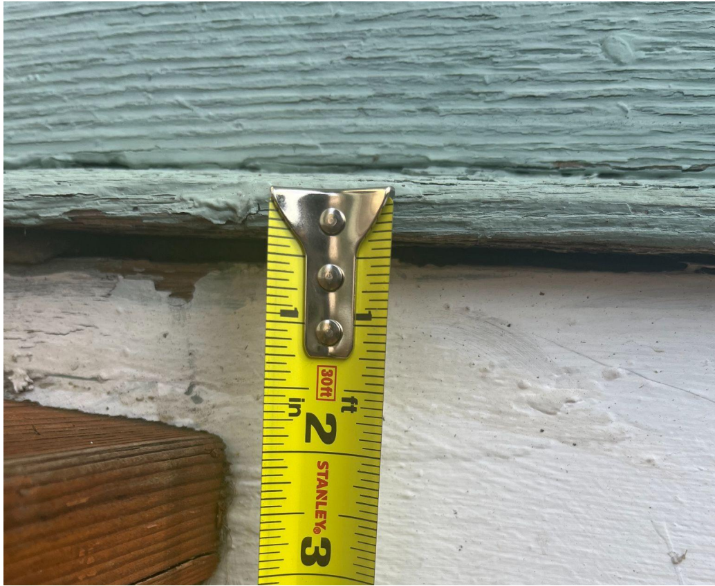
Photo C: Exterior wall of kitchen, gap into basement, daylight
