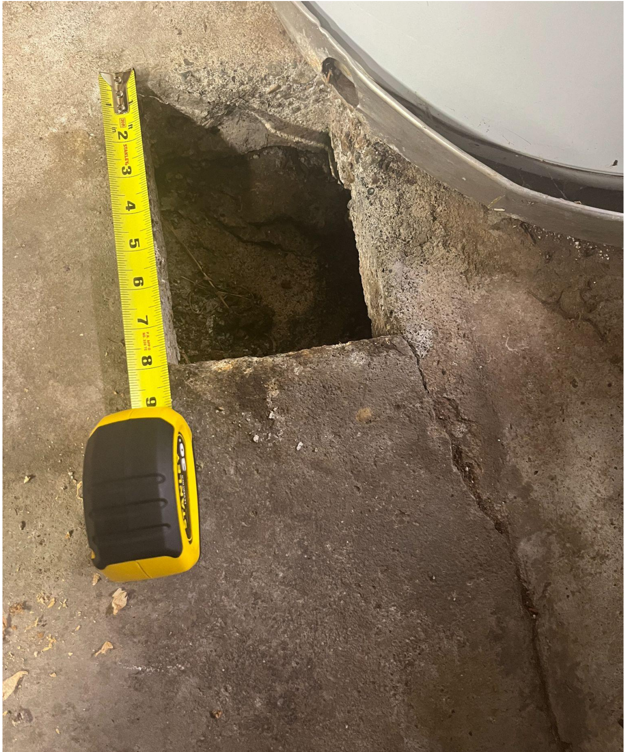
Photo F: Location of missing beam, perhaps removed to put the water heater seen in top right.
