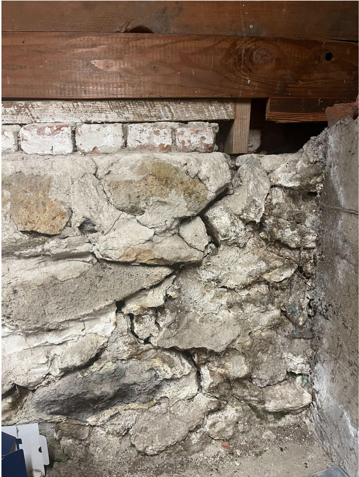
Photo G: Major damage to original foundation, fault line.
