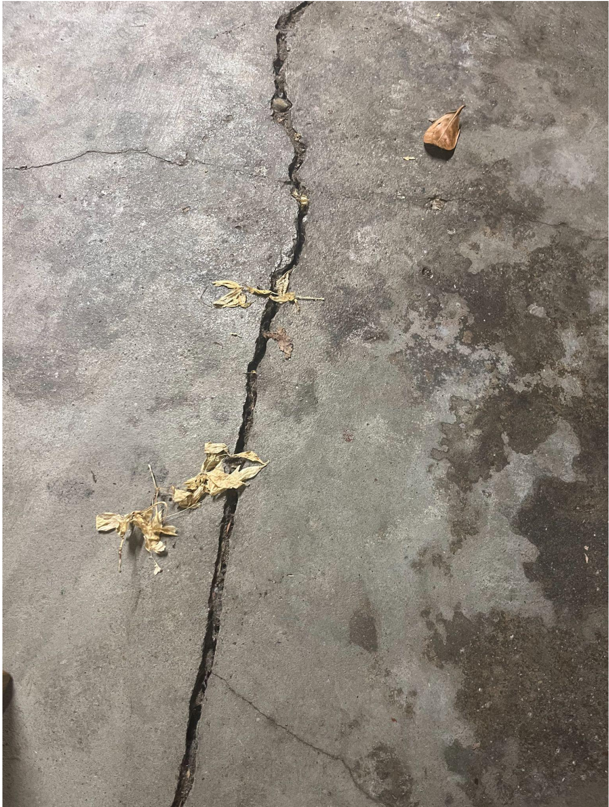
Photo H: Large crack in basement flooring.
