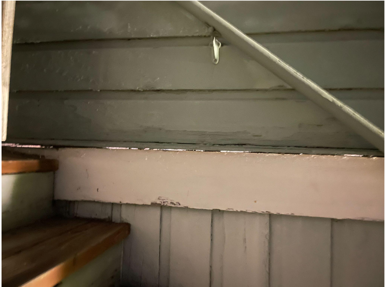
Photo D: Exterior wall of kitchen, gap into basement, night time, seeing basement light.
