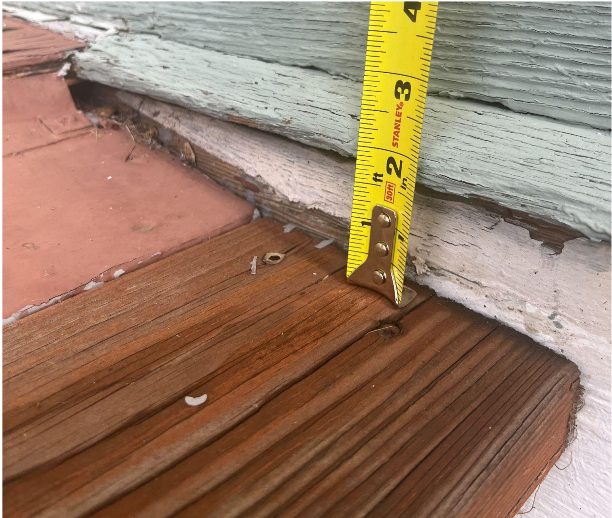
Photo B: Exterior wall of kitchen, paint line
