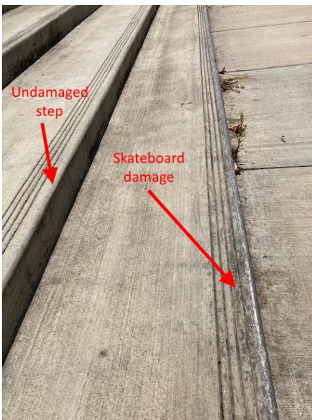
Figure 2 - Skateboard damage on 6th Street steps
