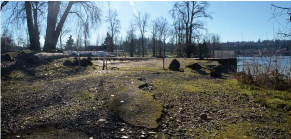
DEGRADED ASPHALT WATERFRONT TRAIL
